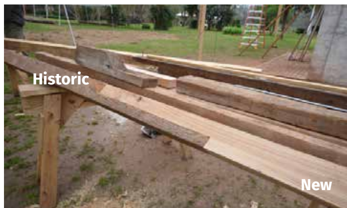
This historic cypress rafter has a new cypress piece sistered in to replace damaged material. The darker wood is the historic material that was retained. Image Credit: NPS|Sarah Marie Jackson.
